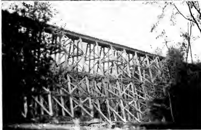
Fig. 1—Steel trestle bridge over Humber River on line of Toronto Suburban Railway.
